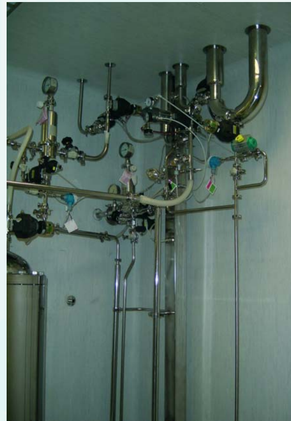
▲ Piping Loop WFI, vapore puro, azoto e scarichi WFI Piping Loop, pure steam, nitrogen and exhausts
