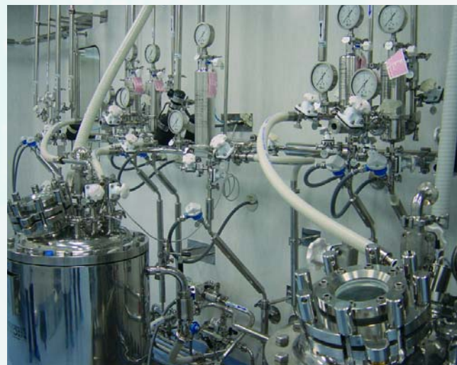
▲ Piping sanitario per sala preparazioni Sanitary Piping for preparation hall
