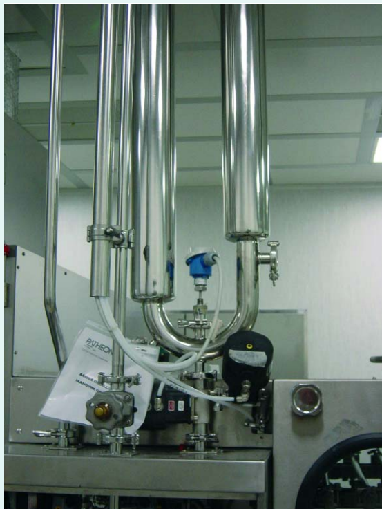
User Point Loop WFI e vapore puro con allaccio alla macchina User Point Loop WFI and pure steam with connection to the machine
