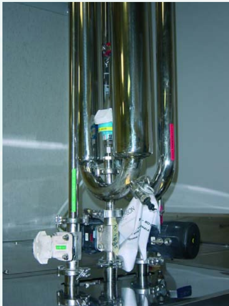
User Point Loop WFI, Loop PW e vapore puro con allaccio alla macchina User Point Loop WFI, Loop PW and pure steam with connection to the machine
